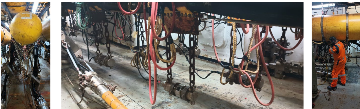
Figure 4.5. A and B) Floats and air guns on deck. C) A mechanic is servicing the air guns.
